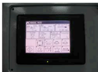
PLC touch screen control
